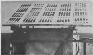
An array of solar cells provides power for a fog signal and obstruction lights on an oil platform in the Gulf of Mexico. The batteries in the container just below the array, operate the equipment at night.
